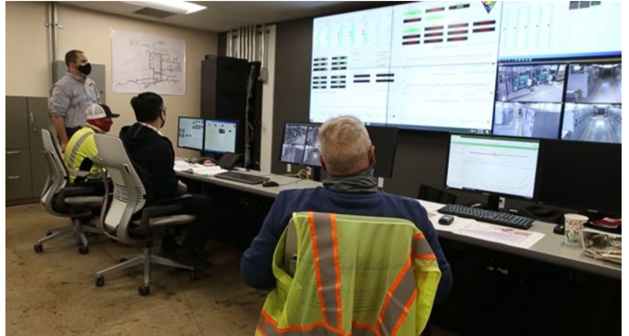
Inside the Energy & Water Operations Center (EWOC) at MCAS Miramar, February 2021
