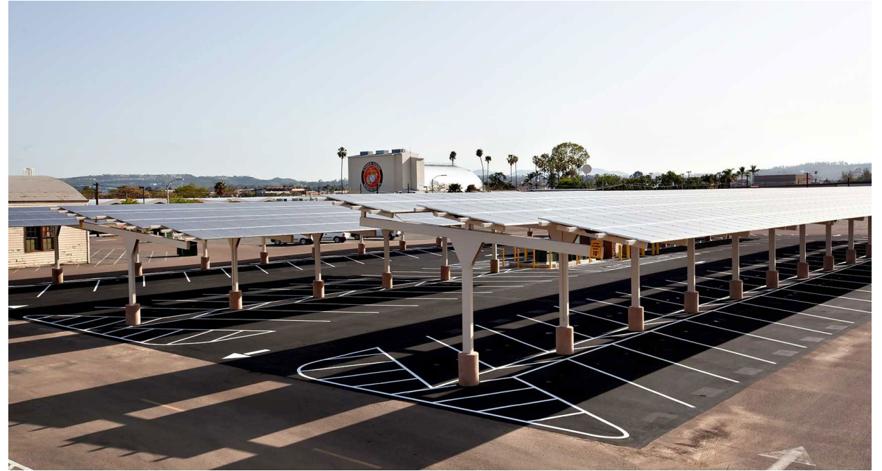
A 250-kilowatt section of distributed solar PV modules serve double duty at MCAS Miramar
