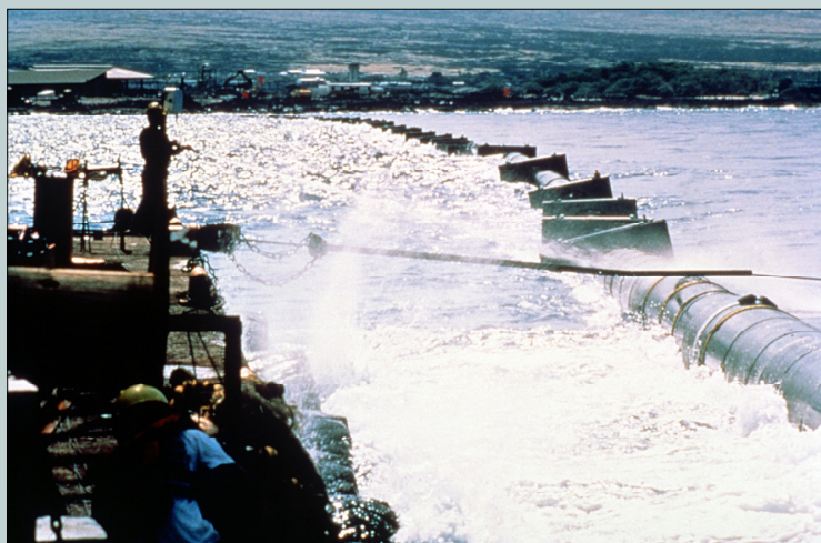
Laying of the cold water pipe at Keahole Point, Hawaii. The pipe supplies the cold water for the OTEC experiment at Hawaii's Natural Energy Lab (Photo by A. Resnick, courtesy of NREL/Released)
