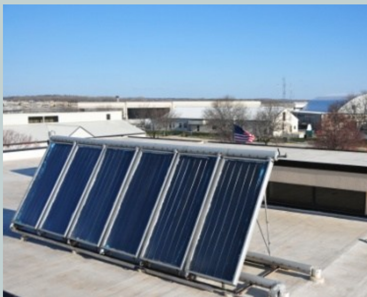
Figure 1. The morning sun hits the solar panels used to preheat water at the 115th Fighter Wing, Wisconsin Air National Guard in Madison, Wis., April 22, 2014. The ANG uses 100 percent green energy. (U.S. Air National Guard photo by 1st Lt. Matthew Wunderlin/Released)
