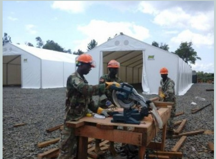
Supporting Operation United Assistance, Armed Forces of Liberia engineers work on the Tubmanburg Ebola treatment unit. Crews quickly put up a series of tents on freshly leveled and graveled ground. The U.S. Agency for International Development is the lead U.S. Government organization for Operation United Assistance. U.S. Africa Command is supporting the effort by providing command and control, logistics, training and engineering assets to contain the Ebola virus outbreak in West African nations. (U.S. Army Africa photo /Released)
