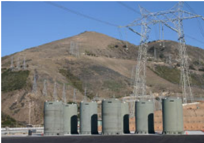
Figure 6-5. Dry Storage Casks [107].
