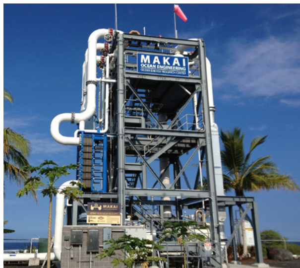
Figure 5-4. The Makai OTEC Plant (Source: Makai Ocean Engineering) [80].
