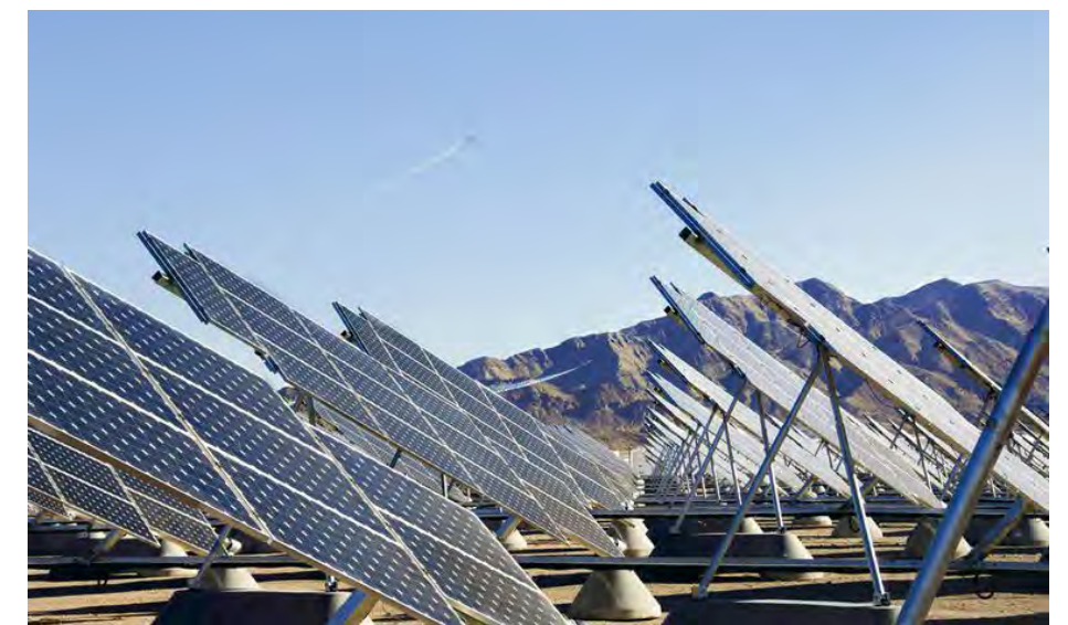
Figure 4: Nellis II, a 19 MW solar PV array at Nellis Air Force Base, Nevada [8]. - (Source: U.S. Air Force photo/150401-F-ZZ999-002)
