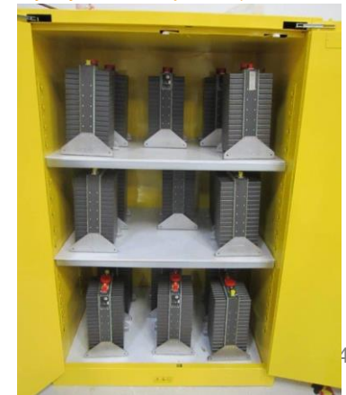
Battery System Ship Set (16 modules)
